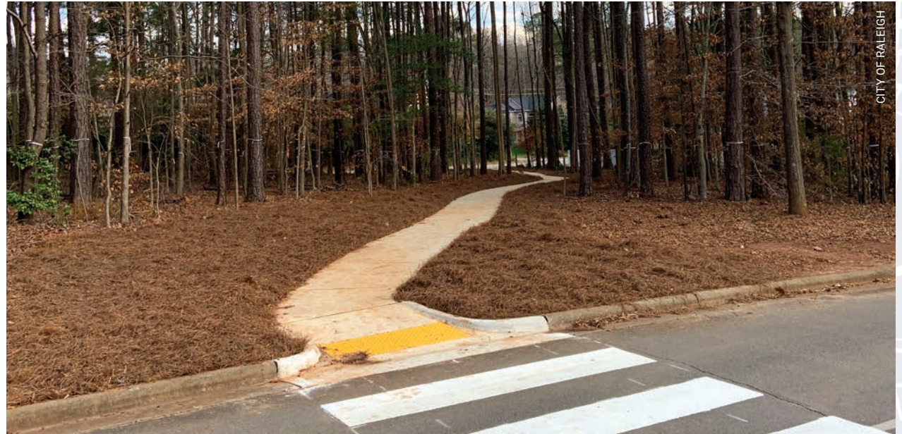
A new sidewalk and crosswalk were installed at Lake Lynn Park to create direct pedestrian access to the park from an adjacent neighborhood. Before this installation, neighborhood residents had to walk along a busy road with no sidewalk—or drive—to reach the park.
