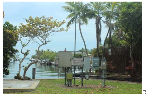
Pumps, pictured here on a waterfront site in the Sans Souci neighborhood, are currently a primary means of dealing with nuisance flooding.
