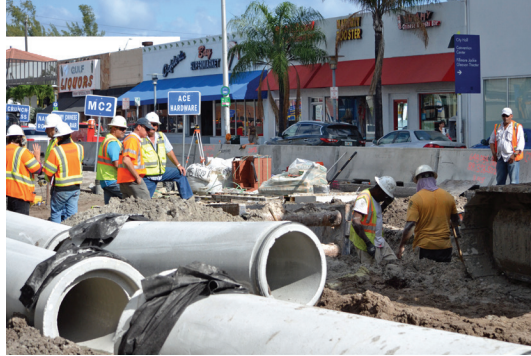
The current program has installed new drainage pipes throughout the city, such as this one on Alton Road.
