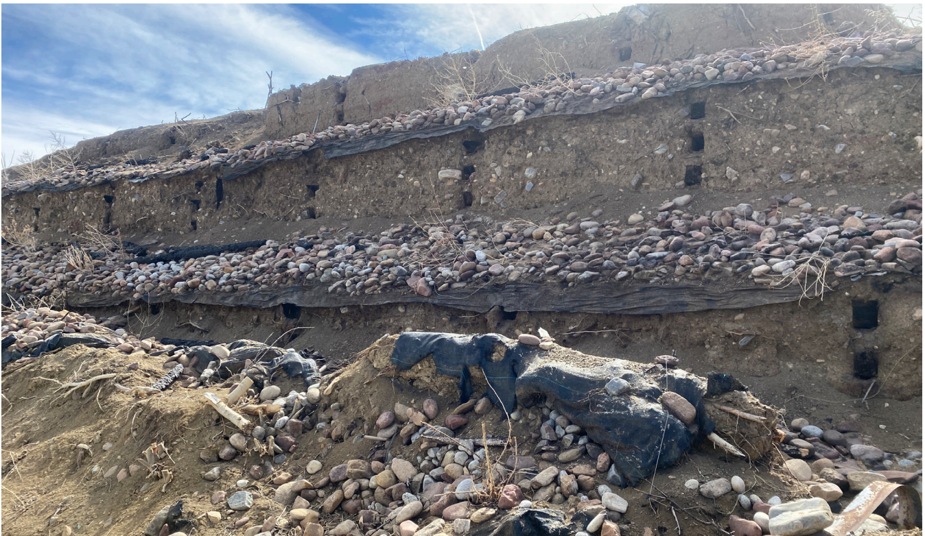
Confusion over responsibility relating to the repair of this retaining wall is delaying surrounding neighbors' ability to rebuild.
