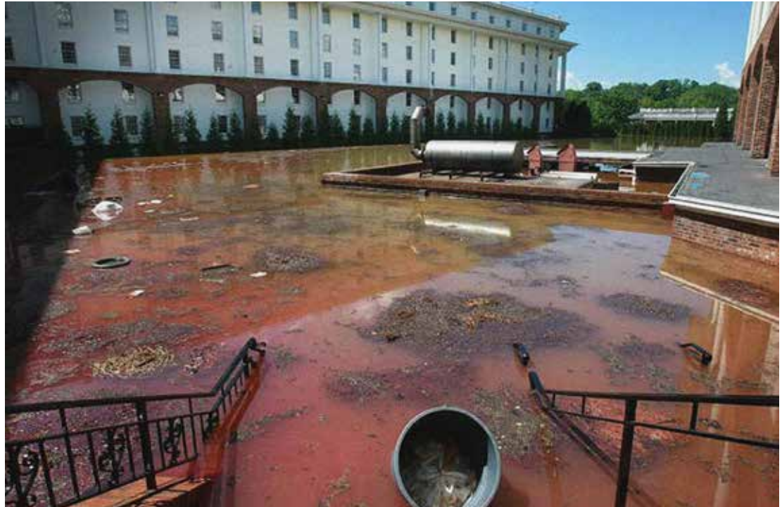
Facility damages stemming from the 2010 floods. The Tennessean
