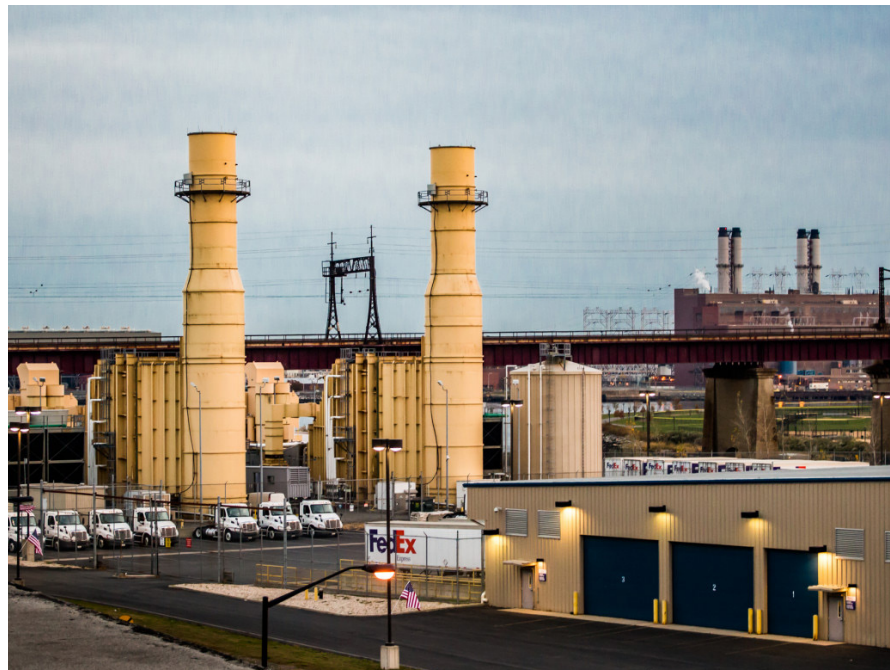
Hell Gate Power Plant, one of many “Peaker Plants” in the New York City area. Source: nylpi.org.
