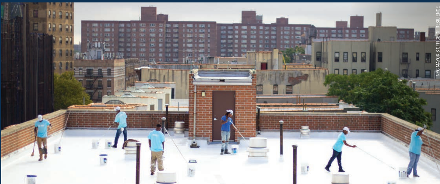
Cool Neighborhoods NYC employs local job seekers to install cool roofs, so the program provides residents with employment and job training as well as helps decrease indoor air temperatures and the need for air conditioning.
