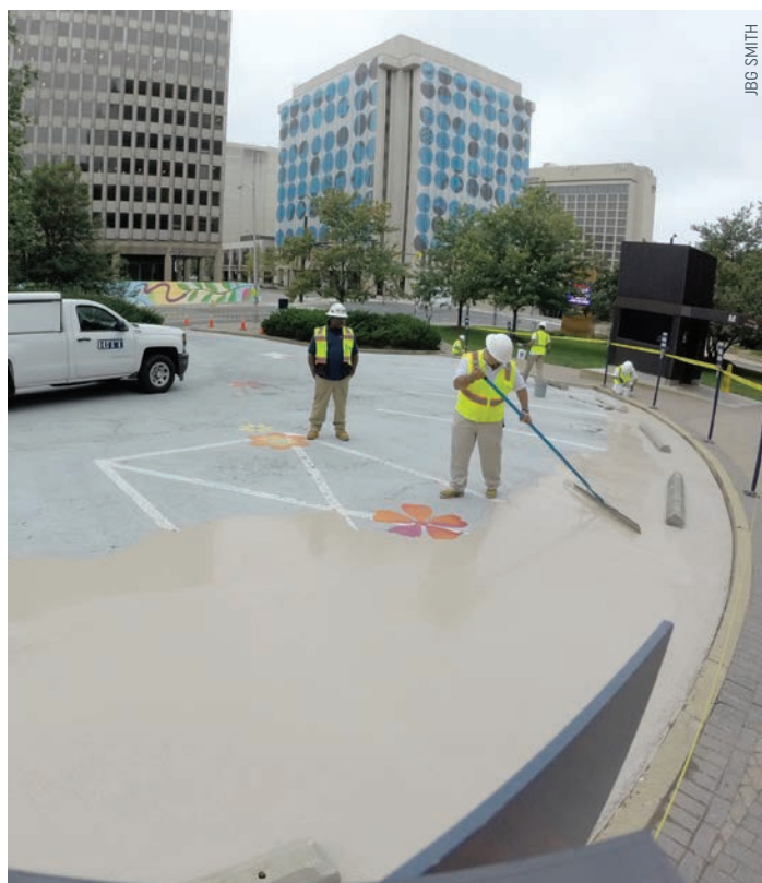
Developer JBG Smith installed 550 gallons of reflective coating over 17,000 square feet and is evaluating the pilot project's outcomes as part of a placemaking strategy.
