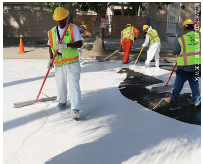
In a city dominated by roads, light-colored, cool pavement may help Los Angeles achieve its ambitious temperature reduction goals.
