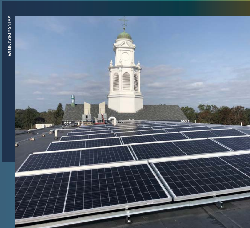
Solar array at The Tyler.
