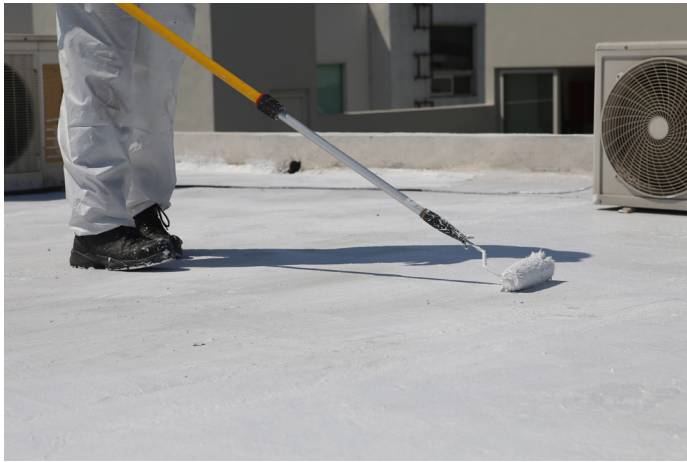
Light-colored coatings can be applied to roofing material to cool a building.
