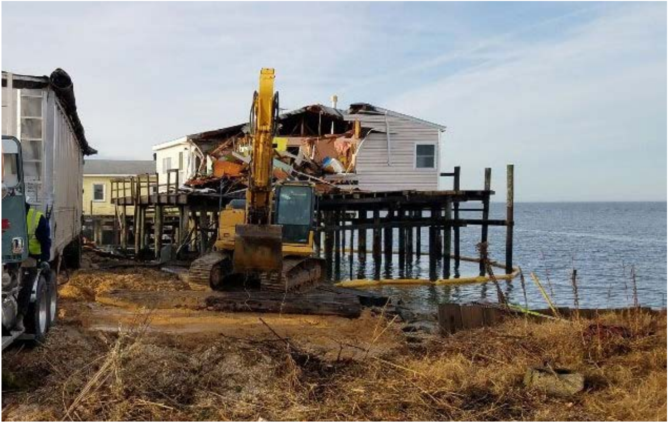
This coastal home in New Jersey is being demolished as part of a buyout in the area, and the land will be returned to support flood absorption.
