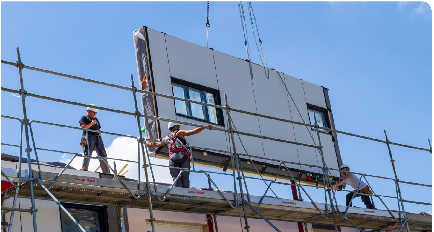
Prefabricated, insulated panels regulate heat and speed up the retrofit process. ( Energiesprong International and Fabrice Singevin )
