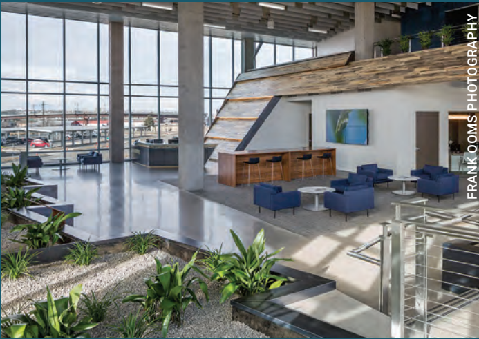
Denver Water headquarters' blackwater is treated on site through various closed and open aerobic tanks, a constructed wetland, as shown in the photo, and a final filtration process before reuse.
