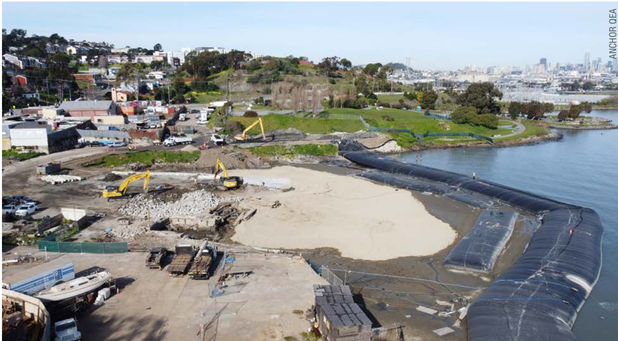
Renovations of three city-owned sites—900 Innes Avenue, India Basin Open Space, and Shoreline Park—are underway and slated for completion in 2026.
