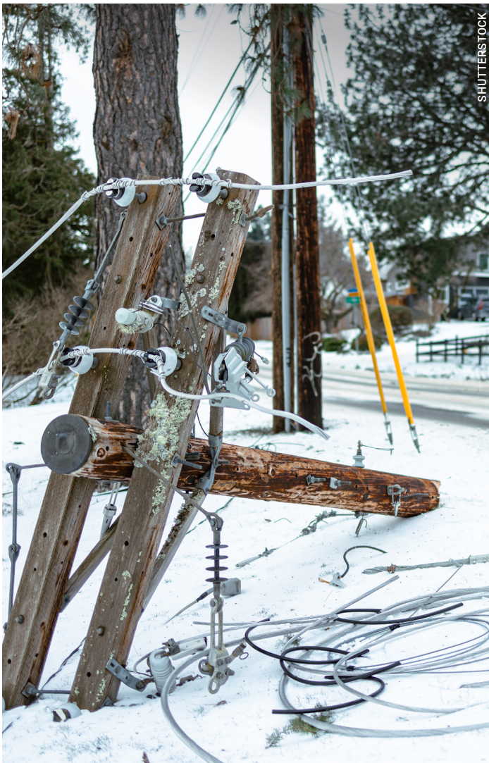
Downed power lines from winter storms can cause outages and disruption to electrical grids.
