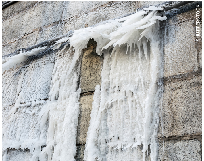
Damage from frozen water after burst pipes can be significant.
