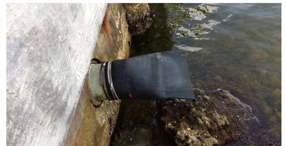
Backflow preventers installed at drainage outfalls in NBV. Photos and plans courtesy of NBV Public Works.
