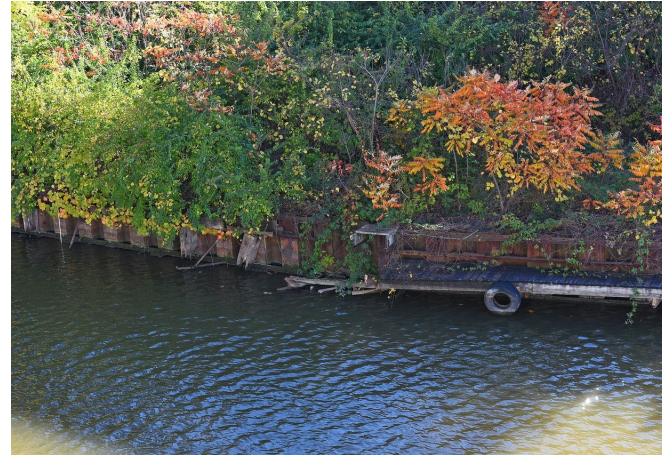
Bulkheads in various states of disrepair along the Cuyahoga River. Many of the bulkheads found along private property were in various states.
