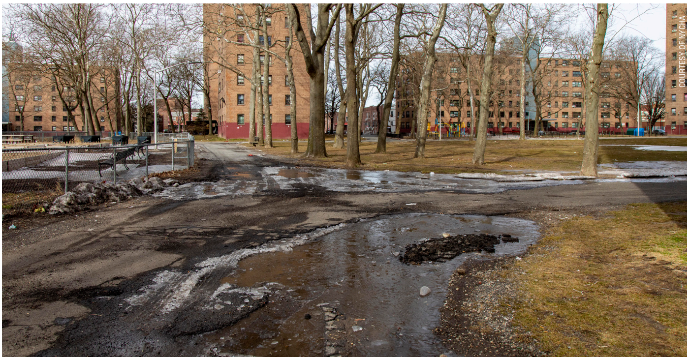
Ponding at Marlboro frequently occurs during rain events.
