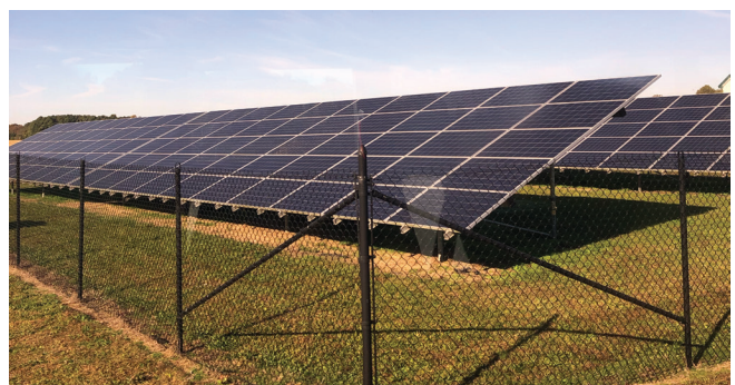
Existing solar panels on the campus
