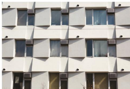
EIFs Insulation wedges with Eco mesh AC units
