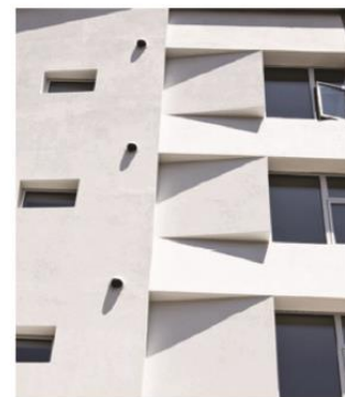
EIFs Insulation wedges with ERV ducts
