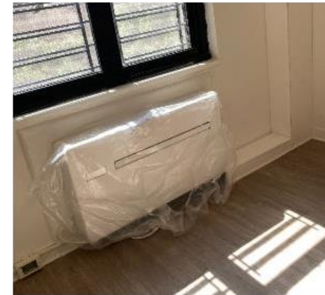
Packaged Terminal Heat Pumps (PTHPs) in each unit
