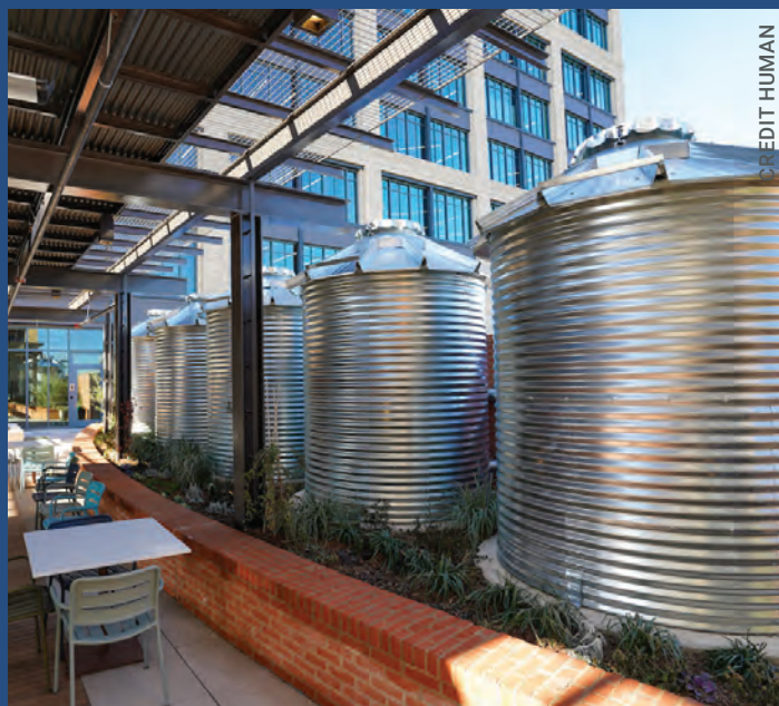
A combination of rainwater capture, storage, and reuse systems make the Credit Human headquarters one of the most water-conscious developments in Texas.
