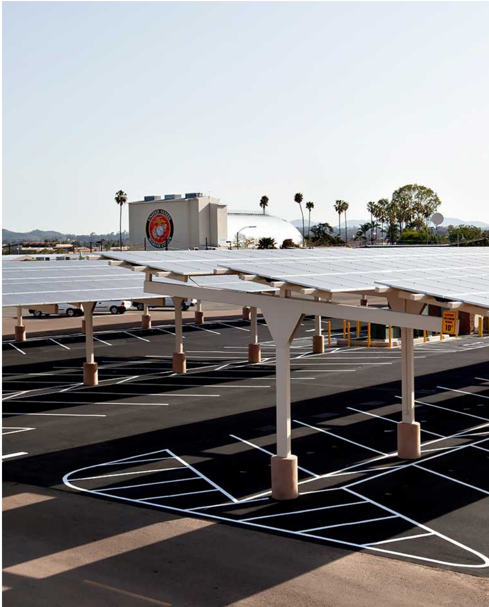
FIGURE 31 As part of its move toward net zero energy, Marine Corps Air Station Miramar installed a 250-kilowatt solar carport in April 2010. ( MCAS Miramar )
