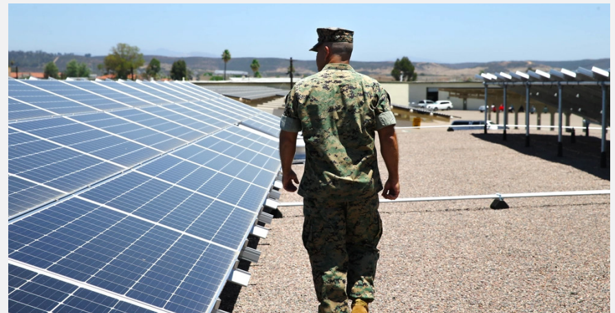
FIGURE 32 A Marine inspects the solar carport at Marine Corps Air Station Miramar. ( MCAS Miramar )
