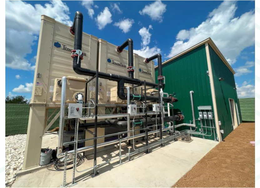
Energy Center 2 – Auxiliary Cooling
