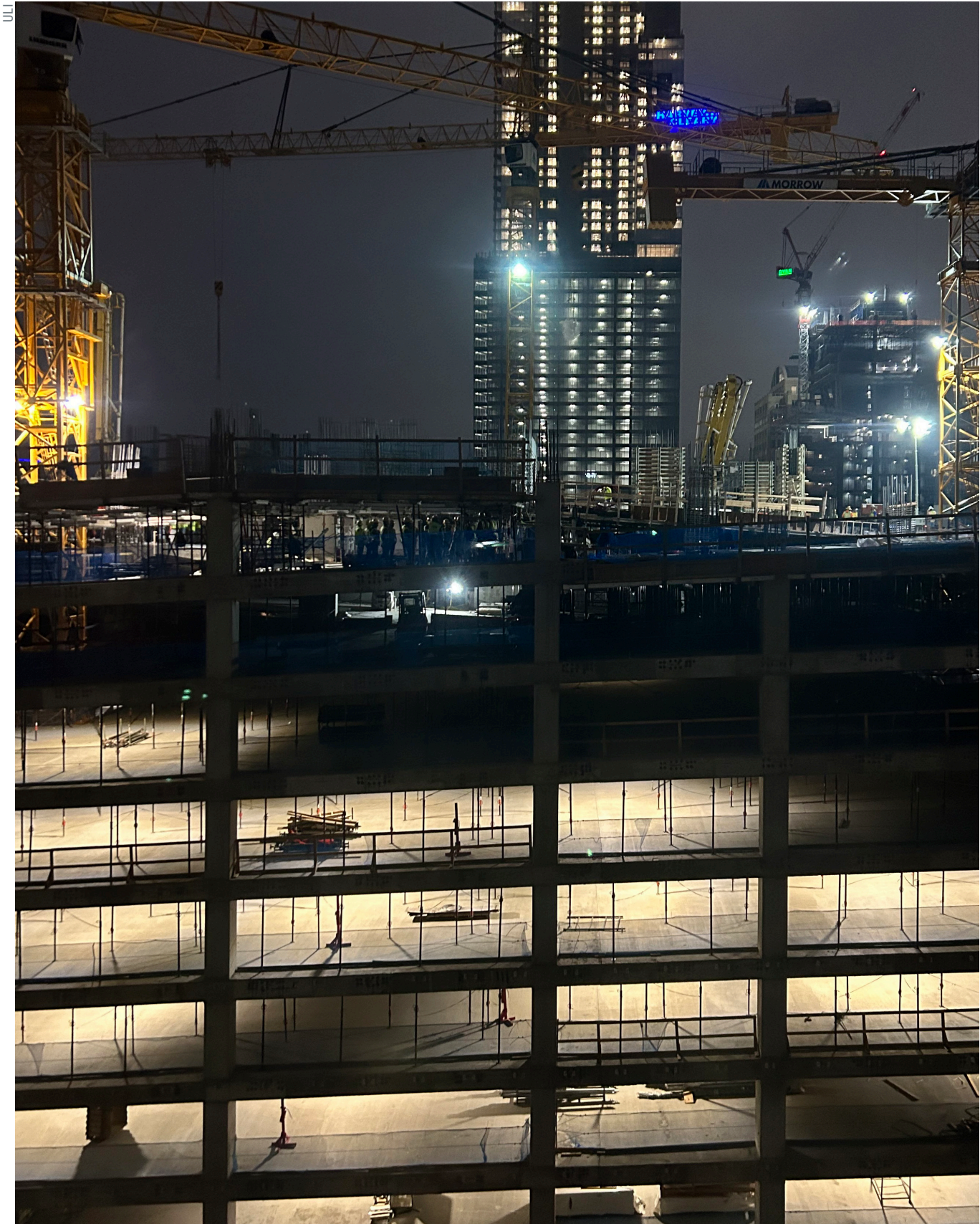
Garage parking under construction in downtown Austin being built to serve the anticipated 20 floors of commercial office above.
